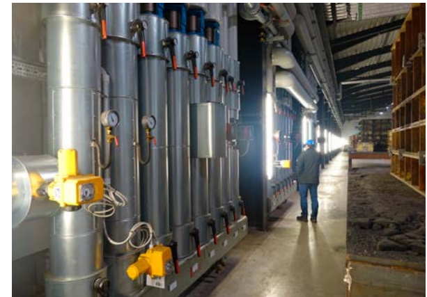
Latest heat recovery plant
