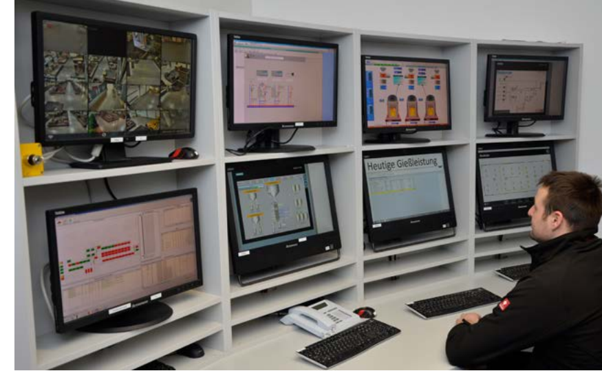
All the processes are centrally monitored at the control station
